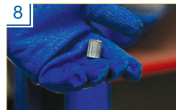
8 Press the small trigger on the shear wrench to eject the bolt spline. The application is now complete.
